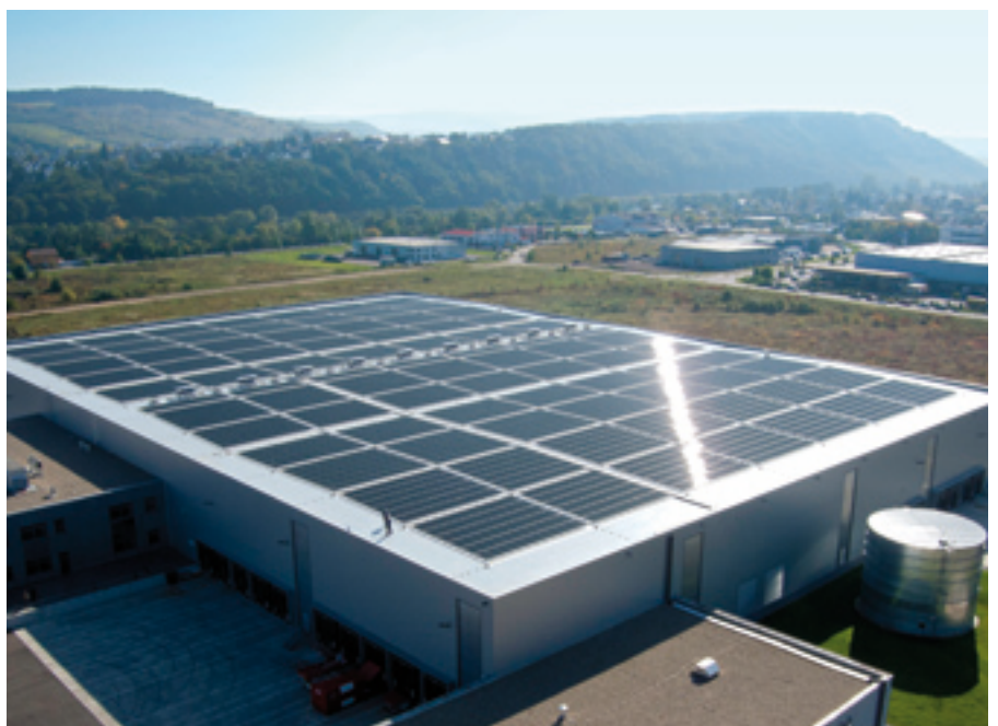
Germany's largest PV system with EVALON® and SOLYNDRA® Solar (Parts Europe, Wasserliesch, Germany)
